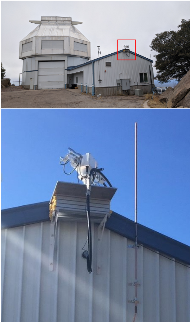
Figure 7. Top: The solar feed assembly installed on its shelf on the end of the WIYN control room building. The weather station to its left is short enough that it does not block the solar telescope’s view of the sky. A new, taller lightning rod has also been installed near the apex of the roof (after this picture was taken—see bottom panel). Bottom: Close-up of the installed solar feed assembly, with the pyrhelimeter and quadrant sensor visible on the left tracker arm. Our optics assembly is on the right arm, behind the body of the tracker. The thick black conduit contains the jacketed solar fiber. Cables are affixed to the back of the tracker to reduce the load on the altitude drives, and wrapped in a tough plastic sheeting to prevent wear from rubbing against the edge of the platform as the tracker rotates. The PVC fitting that routes cables inside the building can be seen directly under the shelf, and the new lightning rod is visible to the right of the solar tracker.
